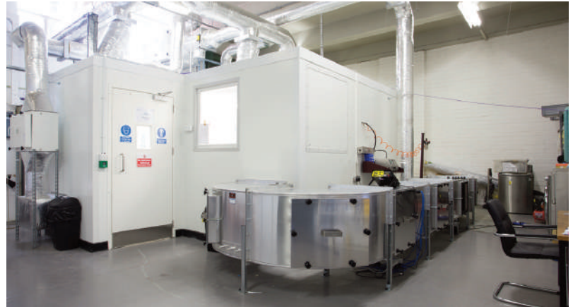
Our test duct rig system (ASHRAE 52.2 modified) attached to a large AHAM type chamber.
